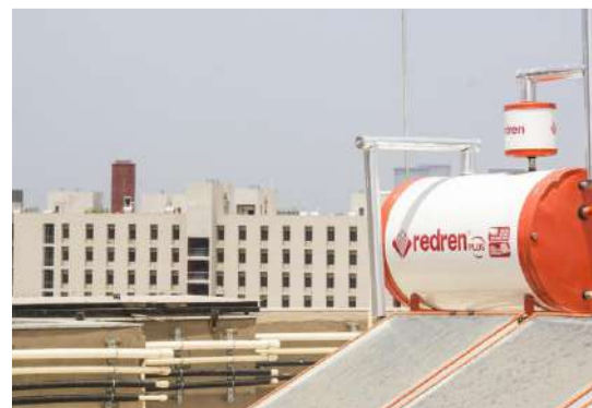
b) Housing solar water heaters
