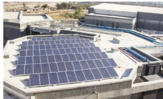
a) Academic building PV panels
